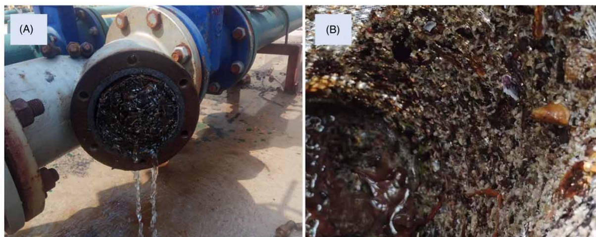
Figure 2 | The fouling problems of water pipes caused by Limnoperna fortunei .
