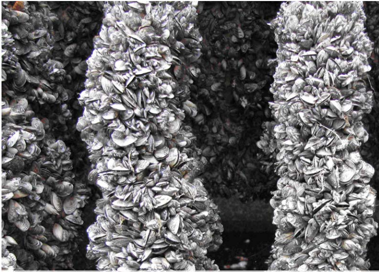
Quagga mussels on intake trashracks at Hoover Dam.
